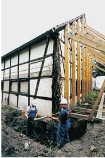
Conversion work on the old stable of the Lahrshof (Source: Bismarck/Schalke-Nord District Bureau)
